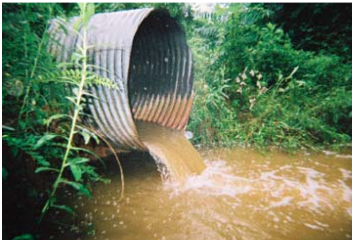
Figure 9. A typical pipe culvert with a drop to the tailwater surface (Camp Creek, Lumpkin County). Photo by Heidi Millington.
